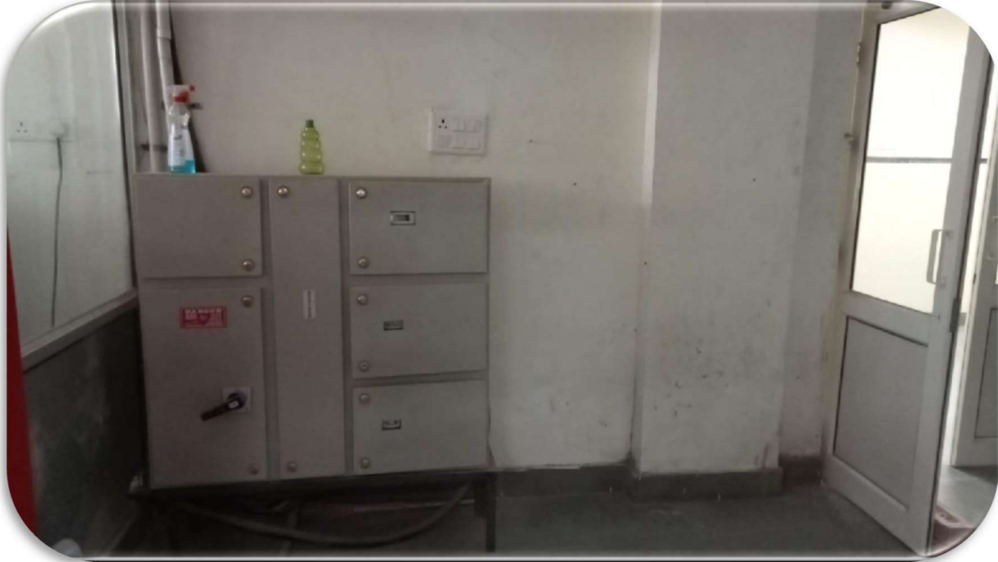
Location for AMF Panel (at First floor):
